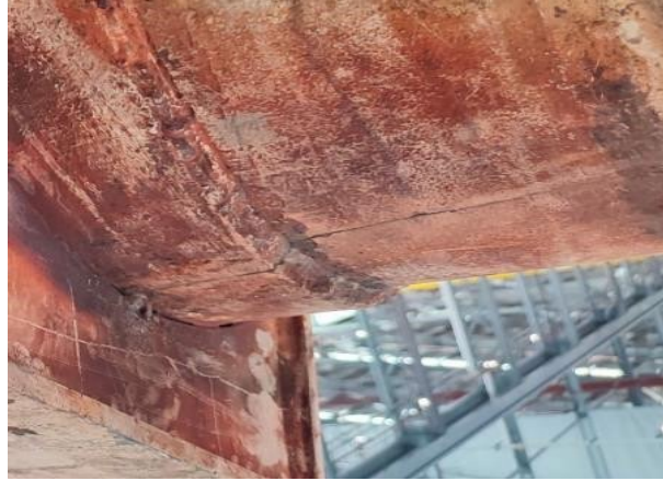
Figure 36.1: Longitudinal and Circumferential Cracks at Saddle Pad to Pipe Fillet Weld
